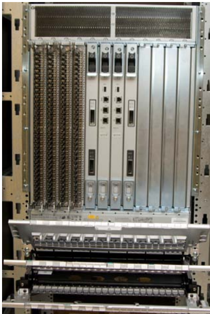
Figure 8. Installed patch panels (below cable comb)
